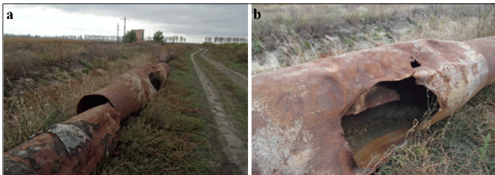
Fig. 4. Condition of the main pipe (Dn 600 steel) at SPP Oțetoaia, year 2019, Vaslui county a - section of pipe replaced; b - detail regarding the structural degradation of the steel pipe (Photo Luca, 2019)
