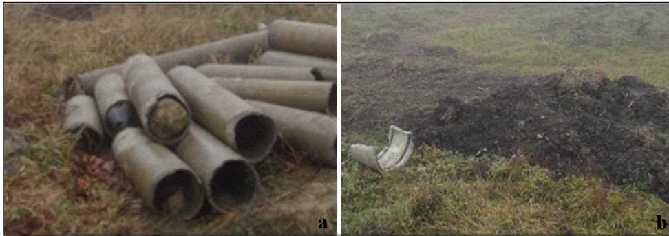
Fig. 5. State of distribution pipes (abasement) from plot SPP16 Berezeni, Vaslui county, year 2015
