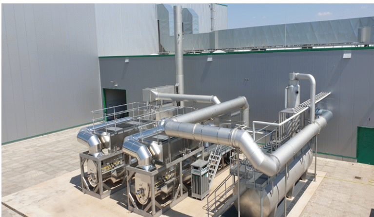
Fig. 2. Installation for capturing, filtering and washing gases, powders and acid vapors [ https://www.electromec.info ]
