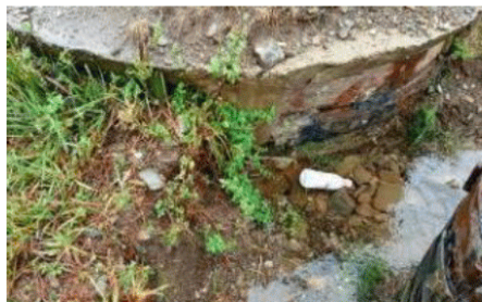
Fig. 5 Confirmation onsite of the water loss
