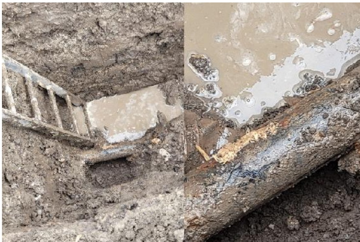
Fig. 3. Identified pipe and loss
