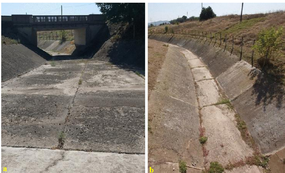
Fig. 5. The state of the flow section of the high flow evacuator a - connection channel (CL); b - inclined drop (CR1) (Luca et al., 2009).
