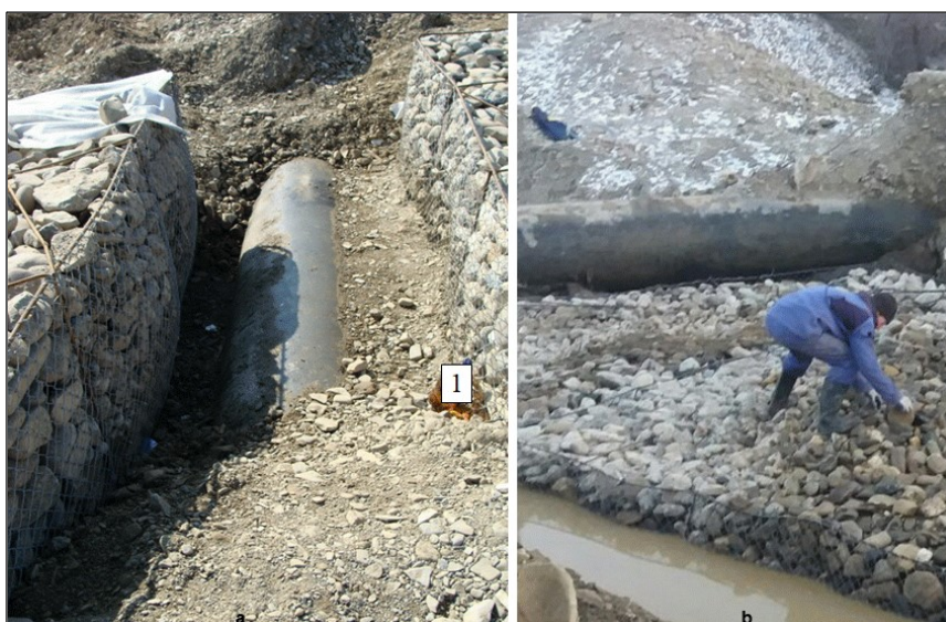
Fig. 7. Protection works on the adduction pipeline located in the shore area of the Tazlaur Sarat river: a – fixing the pipeline to the shore with gabions filled with stone (1 – the location conditions of the pipeline); b – fixing the pipeline in the river bed in the shore area (Luca, 2017)
