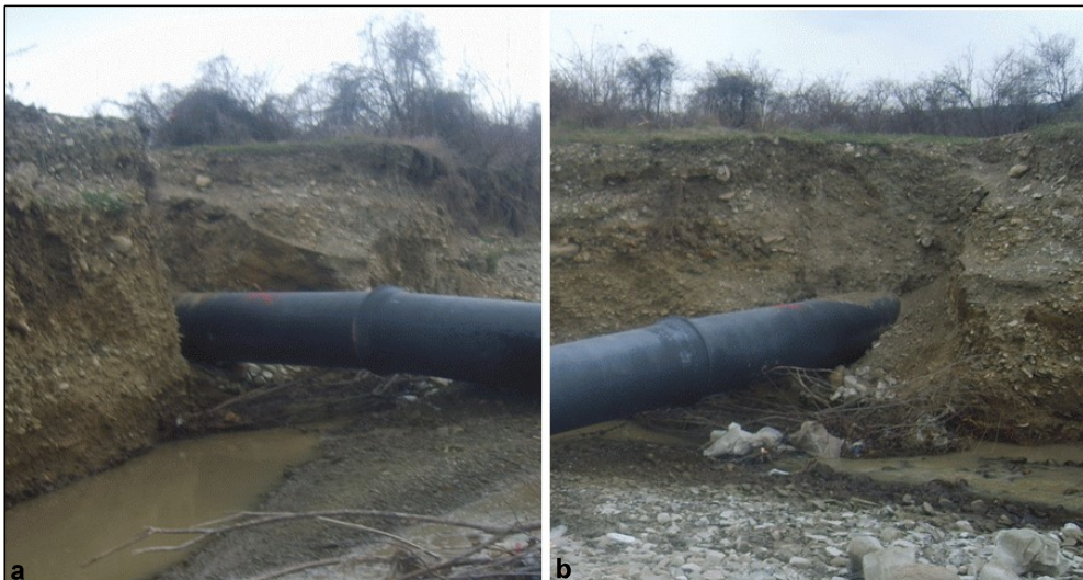
Fig. 6. Bank erosion on the Tazlaur Sarat River in June 2016, with the advance on the bank and the suspension of the adduction pipeline in the Moinesti area: a – downstream view; b – upstream view (Luca, 2017)
