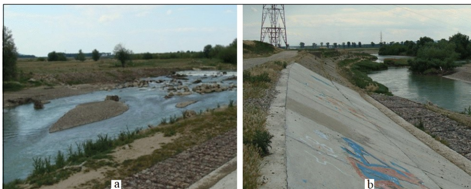
Fig. 5. Moldova River bed interaction - riparian area: a - condition of the bed in the area of the water catchment construction; b – the state of the riparian area, the left bank protection and the downstream catchment bed (photo Luca M., 2020)
