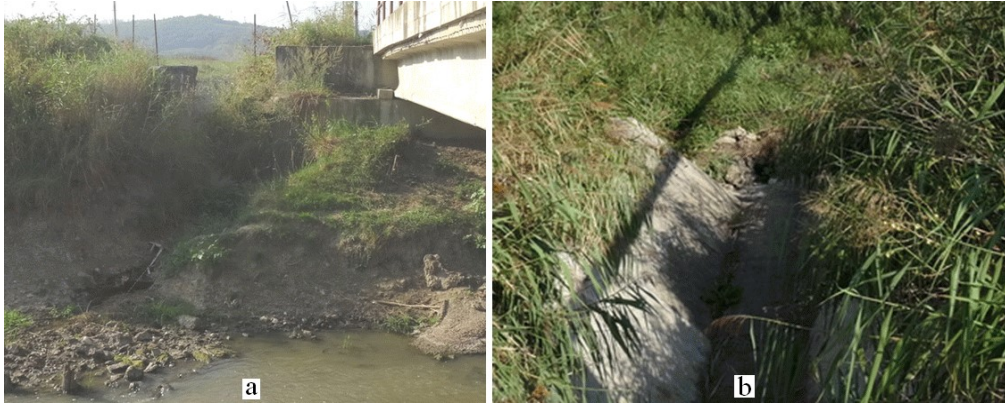
Fig. 7. Bahlui River bed interaction – right bank riparian zone: a – bank erosion by the degraded state of DC4; b – the degradation state of DC1 (Luca M., 2019).
