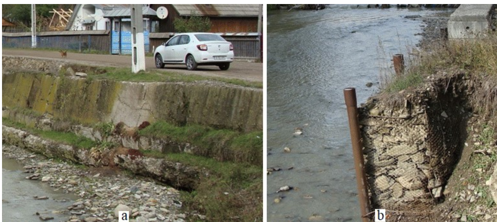
Fig. 2. Tazlăul Sarat River bed interaction - riparian area: a - degradation of the bed and the county road, Chiosa area; b – the degradation of the riverbed and the county road in the "Maxim's canton" area (Luca M., 2016)
