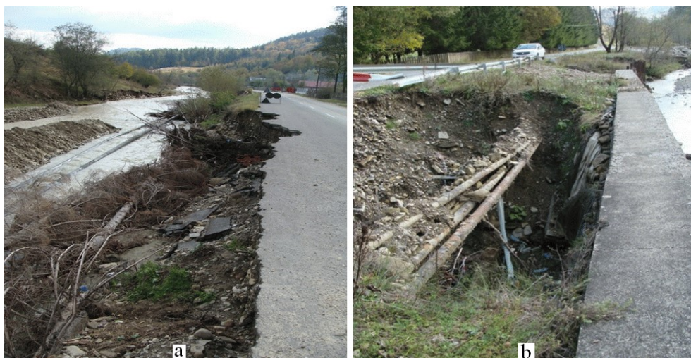
Fig. 3 Tazlăul Sarat River bed interaction - riparian area: a - degradation of the bed and the county road, Chiosa area; b – the degradation of the riverbed and the county road in the "Maxim's canton" area (Luca M., 2016)
